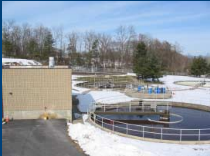
Shippensburg Wastewater Facilities
